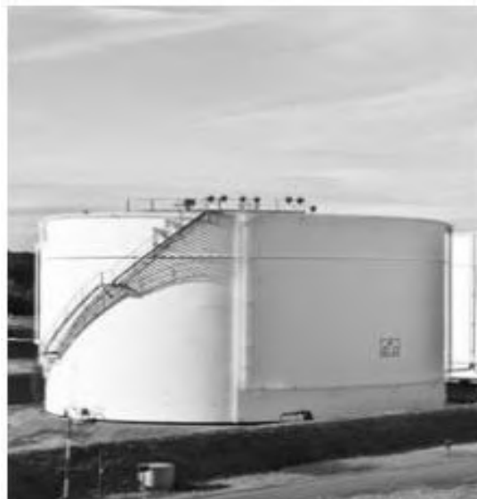
Figure 7.13: Downstream Storage Tank
